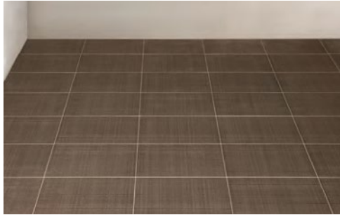
1. Check that the installation screed or existing flooring is clean and flat.
